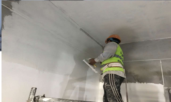
Project Name: MURATA G FACTORY Location: Da Nang Customer: Toda Vietnam Completed: On-Going Scope of Work: Texcoat Exterior & Interior EP
