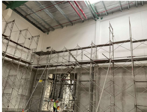
Project Name: KEY TECHNOLOGY FACTORY Location: Vinh Phuc Customer: Toda Vietnam Completed: On-Going Scope of Work: EP Painting Work
